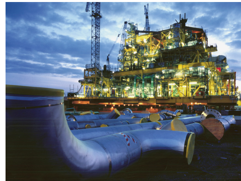
Brent Charlie replacement modules during final onshore commissioning for the Brent Field refurbishment programme
